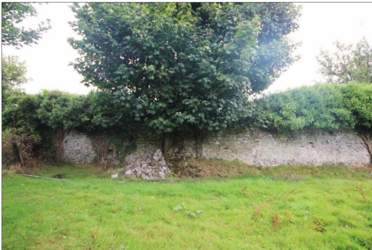
Plate 77: Section of collapse in western wall
