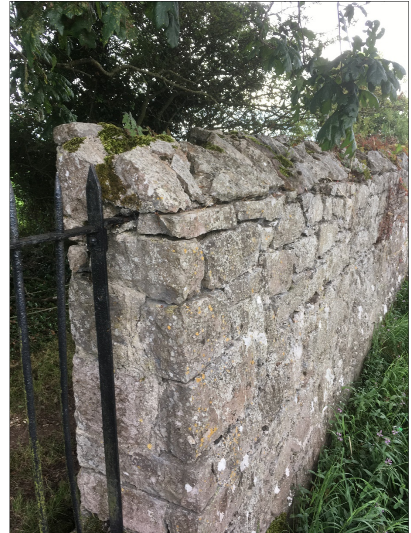
Figure 3: Example of constructed masonry capping to historic rubble limestone wall. A slight overhang of capping beyond the vertical surface of the wall of approximately 30mm has proven to significantly reduce the effects of weathering on historic masonry walls.
