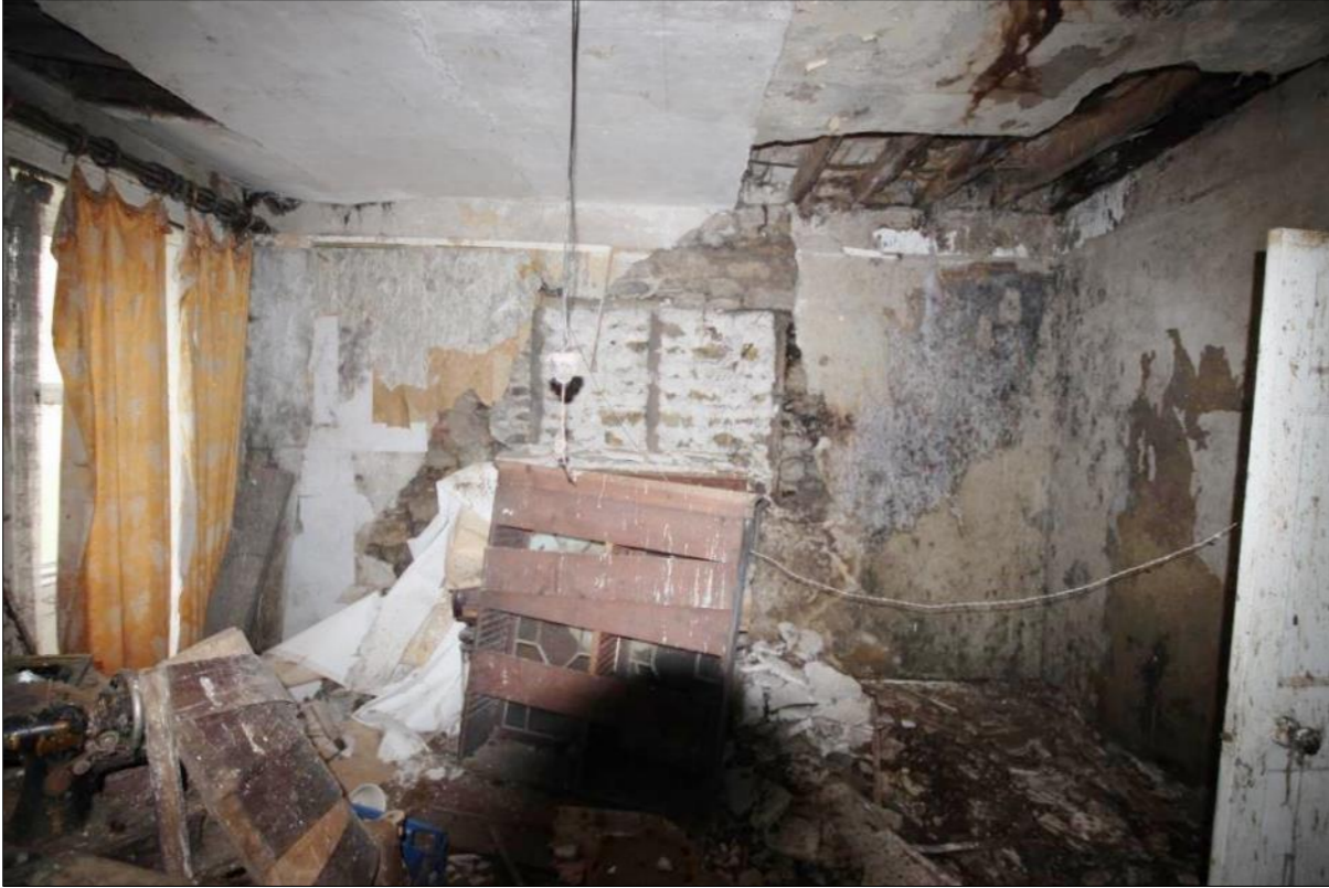
Plate 39: Ground floor room GF02 looking towards return with possible blocked up opening
