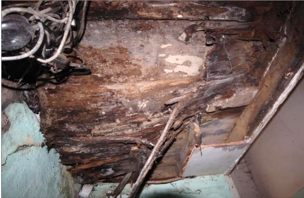
Plate 46: Decayed floor in hallway under stairs
