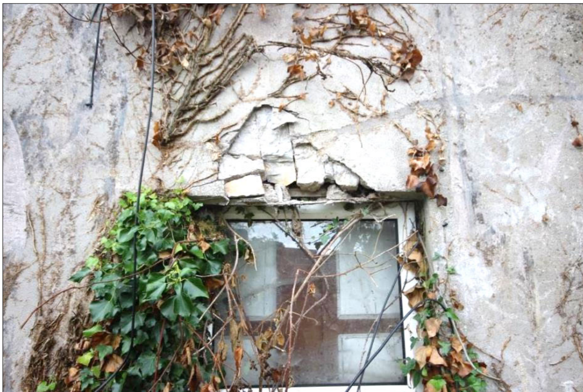
Plate 33: Deteriorating render on rear elevation
