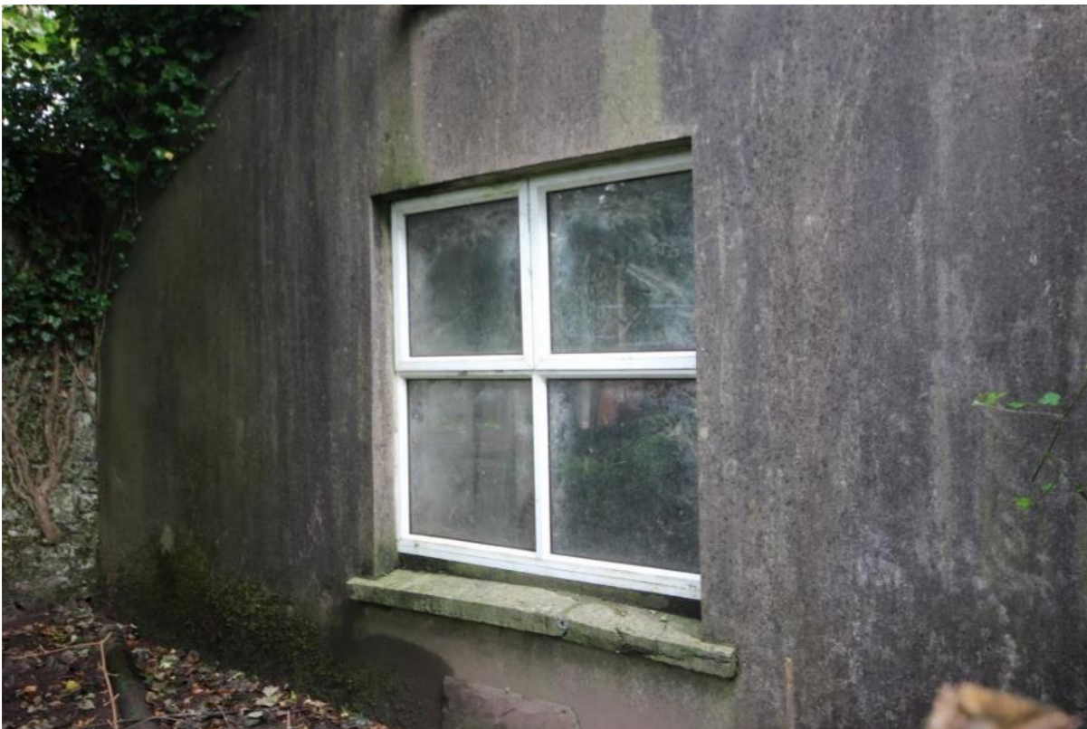
Plate 36: Front elevation with altered window cill and uPVC window
