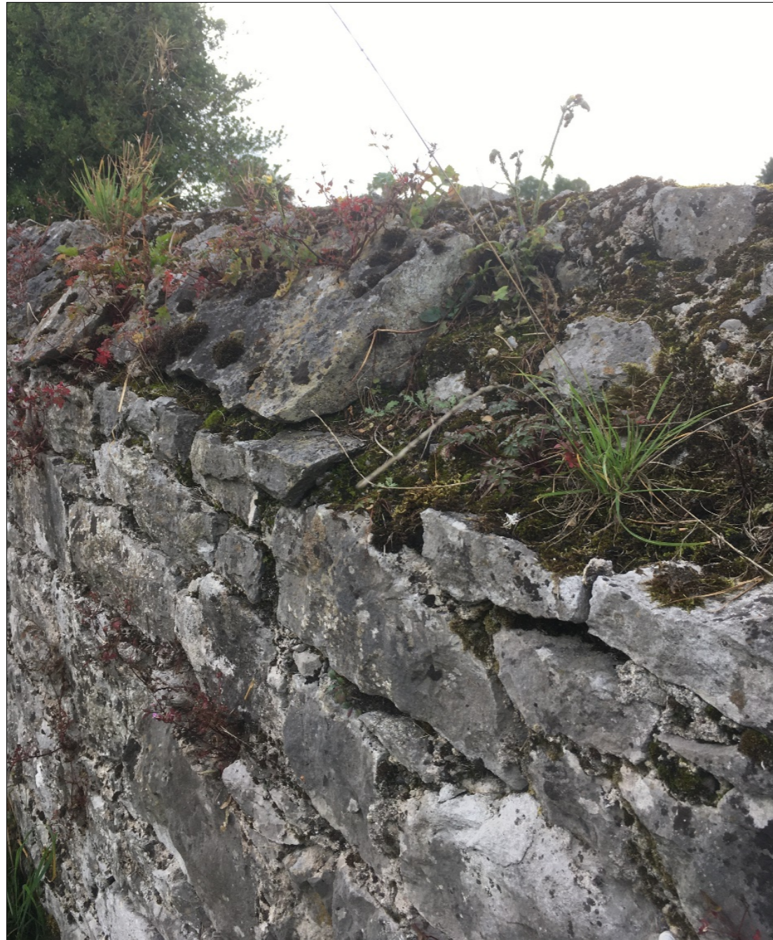
Figure 2: Example of constructed masonry capping to historic rubble limestone wall with sloped top surface built of triangular-shaped stones. Example shows weathered masonry, but joints should all be pointed flush with lime mortar to prevent pooling of water on wall-top. Note use of large stones to help tie wall-top faces together and retain stability.
