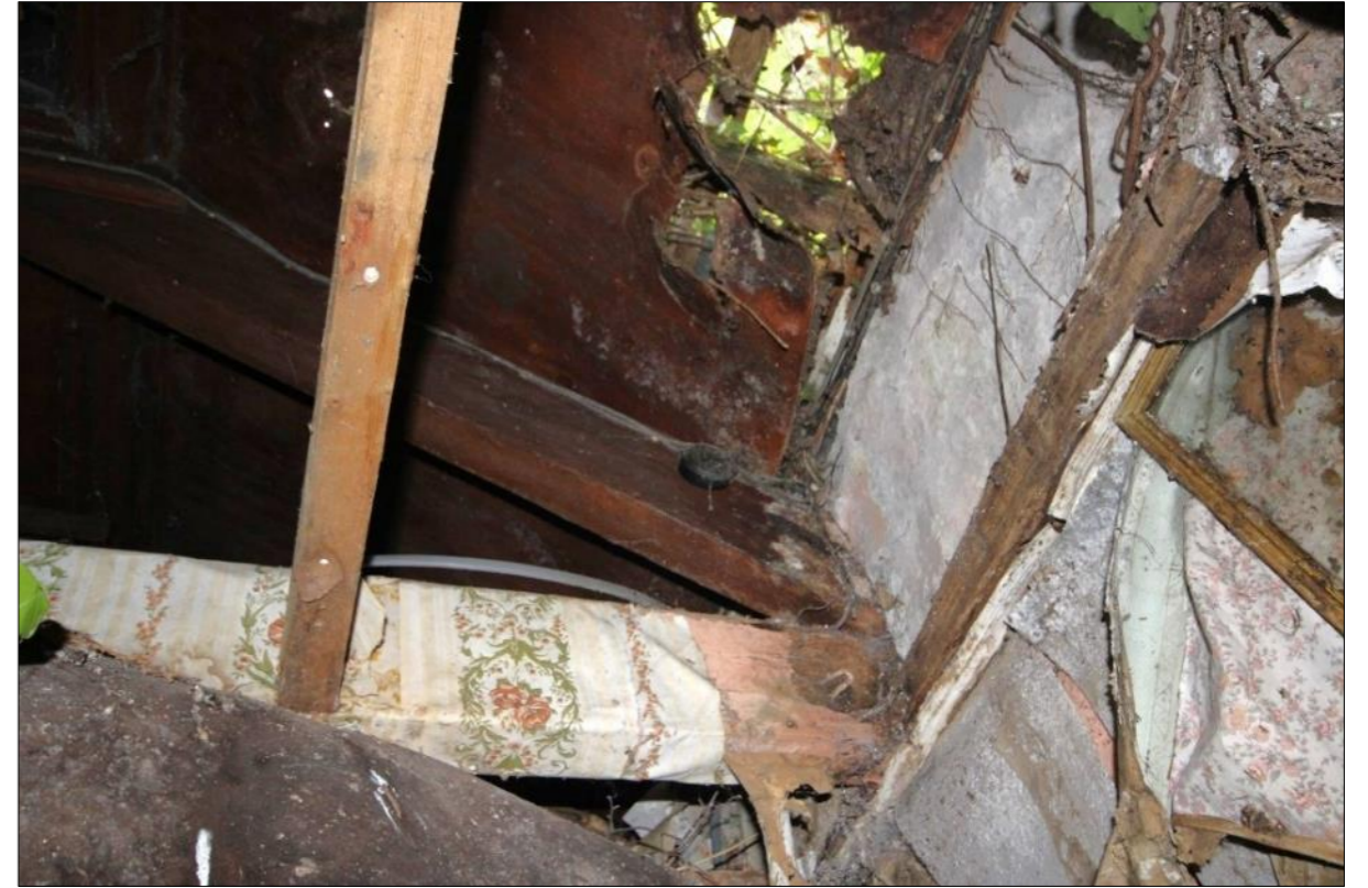
Plate 21: Damaged roof in GF01
